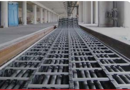
Mobile onshore power supply
